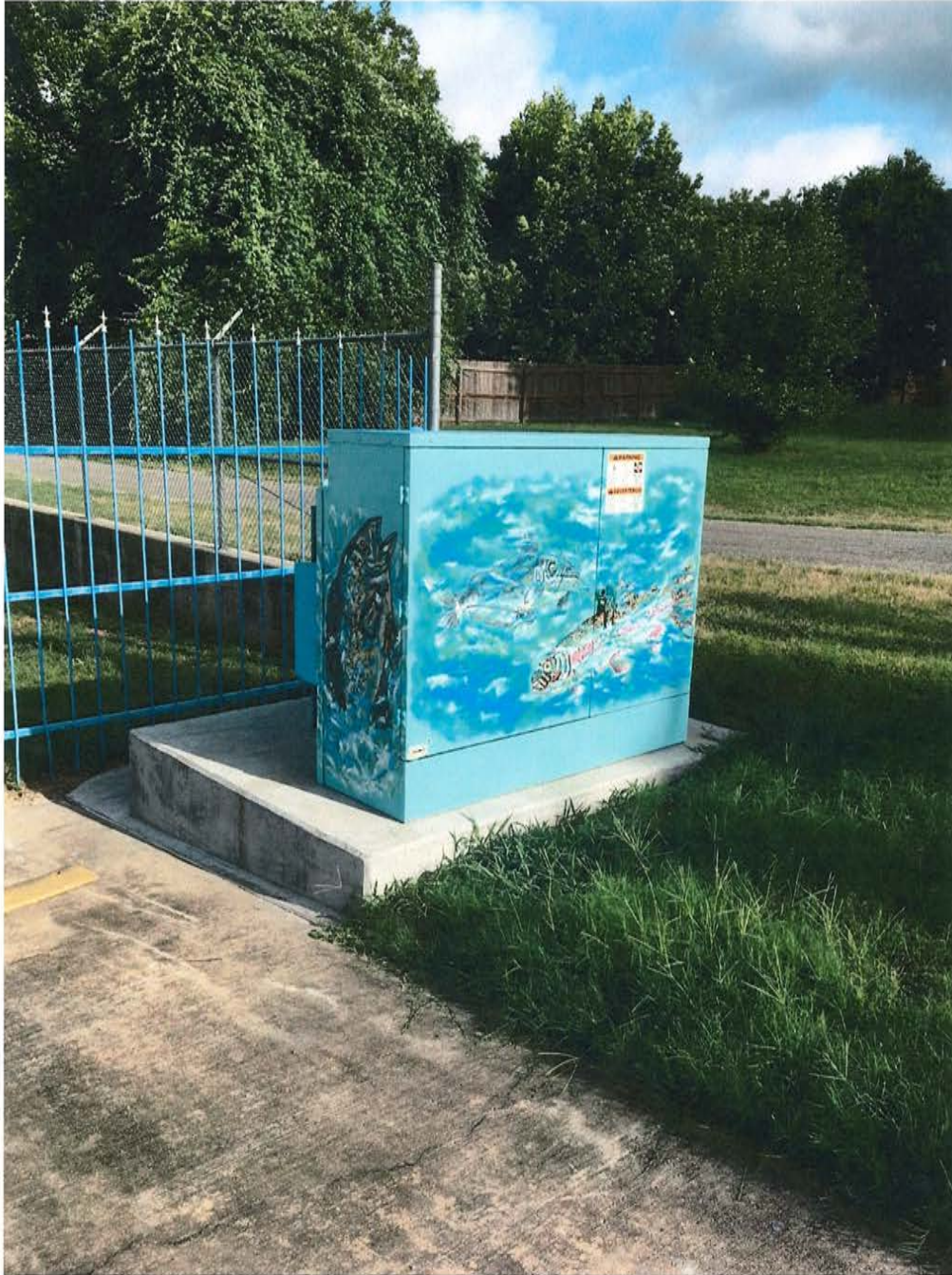
Example of previous Transformer project located at the Willow water treatment facility
